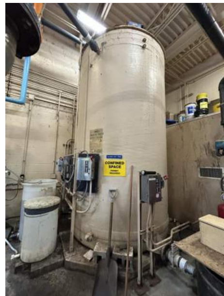
Figure 2-23 Sludge Day Tank
