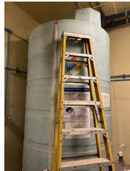
Figure 2-15 Sodium Aluminate Storage
