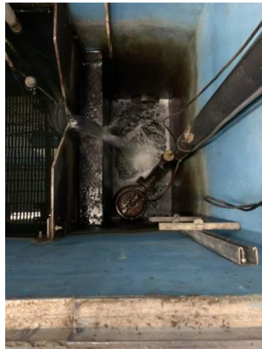
Figure 2-20 Effluent Wet Well & V-Notch
