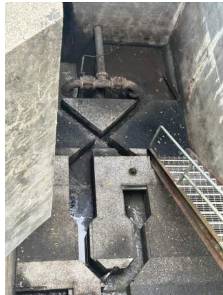
Figure 2-11 Influent Wet Well
