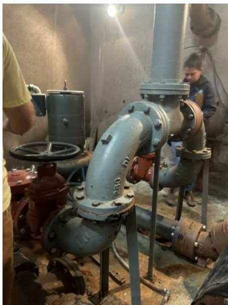
Figure 2-12 Influent Pumping System
