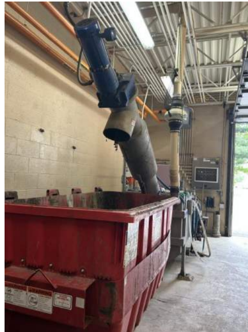
Figure 2-21 Septage Receiving Unit
