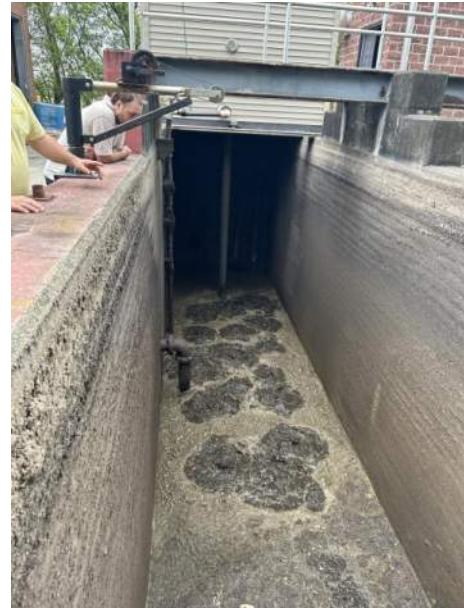
Figure 2-22 Aerobic Sludge Holding Tank
