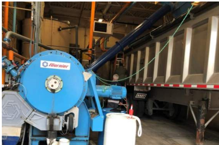
Figure 2-25 Rotary Press Conveyor System
