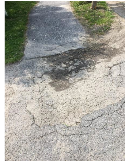
Rough sidewalk and driveway surface
