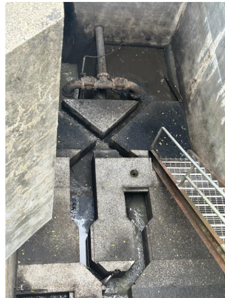
Figure 2-11 Influent Wet Well
