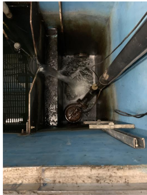
Figure 2-20 Effluent Wet Well & V-Notch
