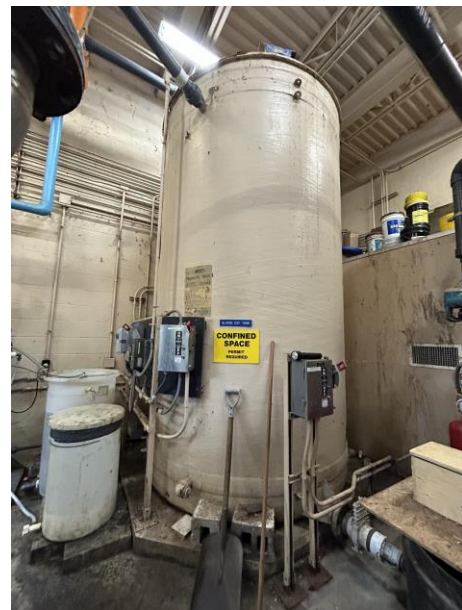
Figure 2-23 Sludge Day Tank
