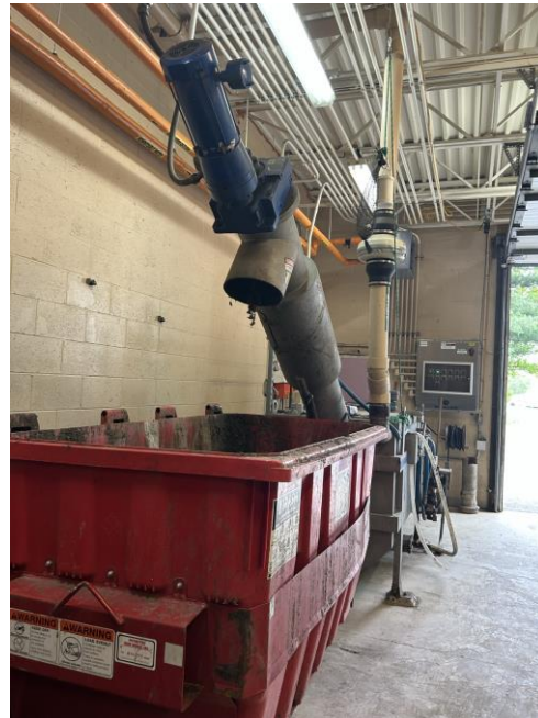
Figure 2-21 Septage Receiving Unit
