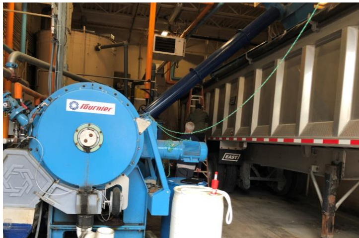
Figure 2-25 Rotary Press Conveyor System
