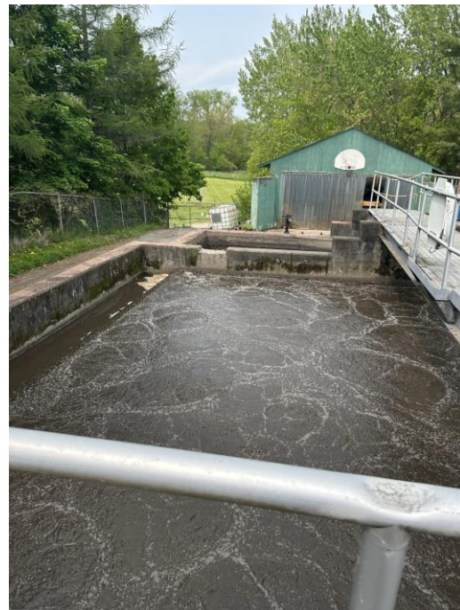
Figure 2-14 Biological Aeration Tank
