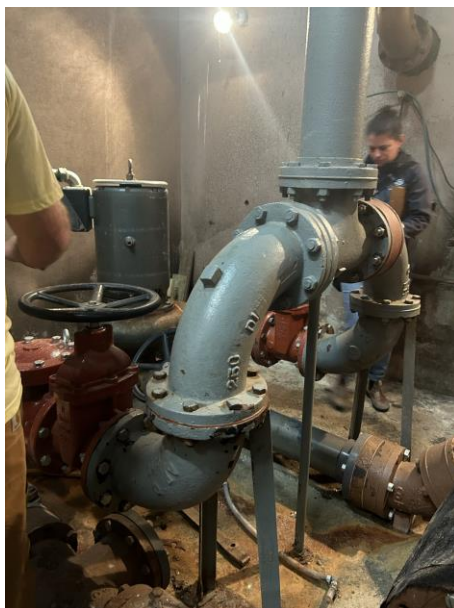
Figure 2-12 Influent Pumping System
