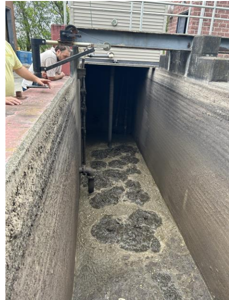
Figure 2-22 Aerobic Sludge Holding Tank
