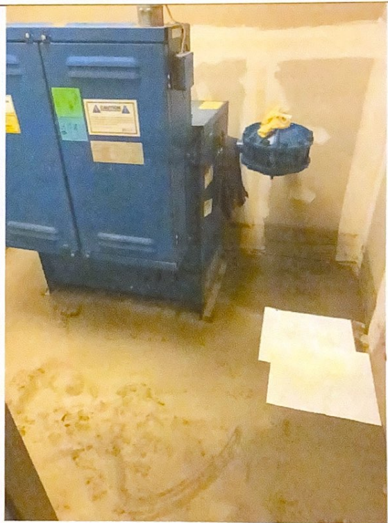
Town Center Basement Elevator Room
