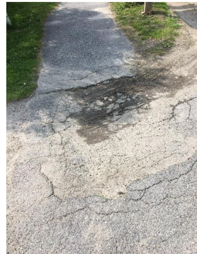
Rough sidewalk and driveway surface
