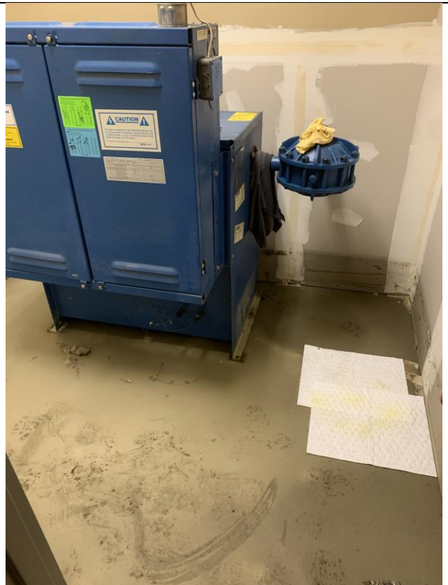
Town Center Basement Elevator Room
