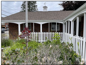
REMOVE PICKETS & INTERMEDIATE FRAMING BETWEEN PORCH SUPPORTS. REPAIR WOOD AS REQUIRED & PAINT
