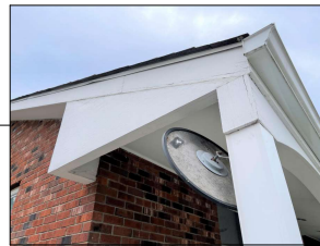
REMOVE EXISTING ROOF RETURNS ON CUSTOMER ENTRANCE PORCH. EXTEND SOFFIT AND ADD NEW ROOF RETURN FLUSH WITH WALL, SAME HEIGHT.
