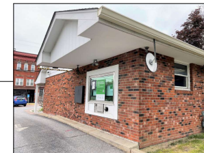
REMOVE EXISTING LIGHTS AT DRIVE-THRU. REPLACE WITH 3 TYPE: PR111L SERIES. LIGHT RECESSED LIGHTS. REPLACE NIGHT DEPOSITORY NEXT TO DRIVE-THRU WINDOW.
