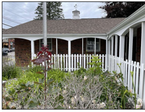
REMOVE PICKETS & INTERMEDIATE FRAMING BETWEEN PORCH SUPPORTS. REPAIR WOOD AS REQUIRED & PAINT
