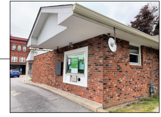
REMOVE EXISTING LIGHTS AT DRIVE-THRU. REPLACE WITH 3 TYPE 'PRISL' SERIES LIGHT RECESSED LIGHTS. REPLACE NIGHT DEPOSITORY NEXT TO DRIVE-THRU WINDOW.
