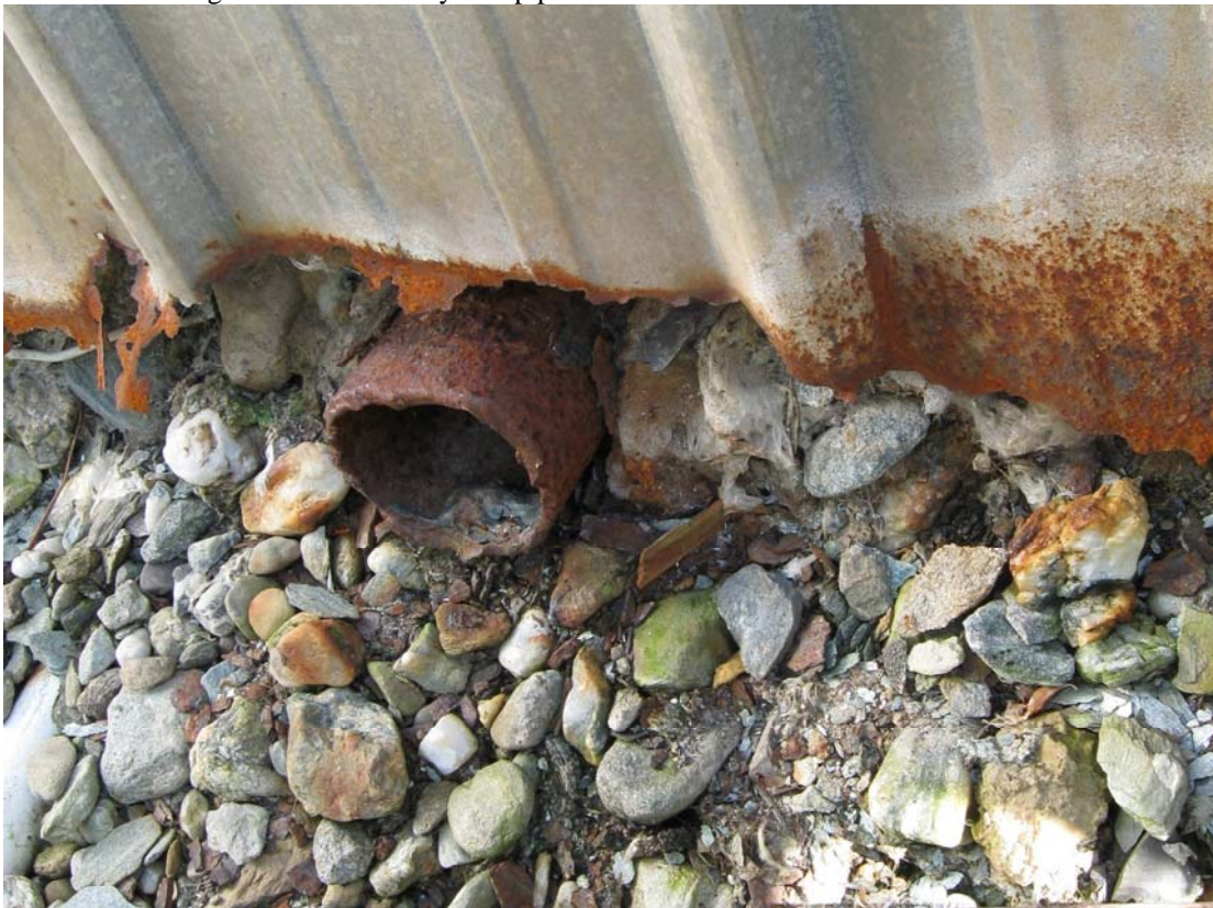
Plate 6: Severed pipe in rear of boiler building
