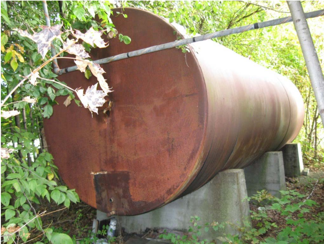
Plate 7: Above ground heating oil storage tank
