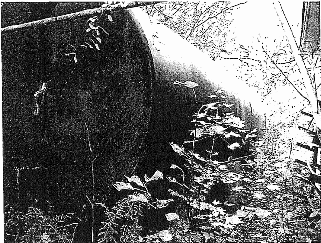
Photo #6: Above ground storage tank.
