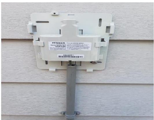
Shows exterior mounted conduit, wall plate and MIU.
