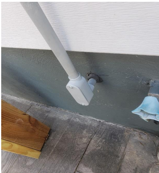
Shows conduit from basement. It contains wires from the MIU.
