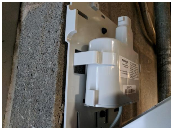
Shows interior mounted wall plate and MIU.
