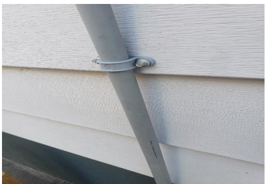
Shows exterior mounted conduit. It contains wires from the MIU.
