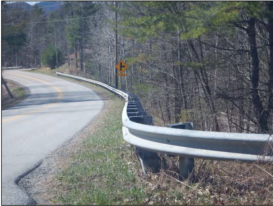
Photo 10. Photo shows the guide rail on the west side of Jericho Road. View is to the south.
