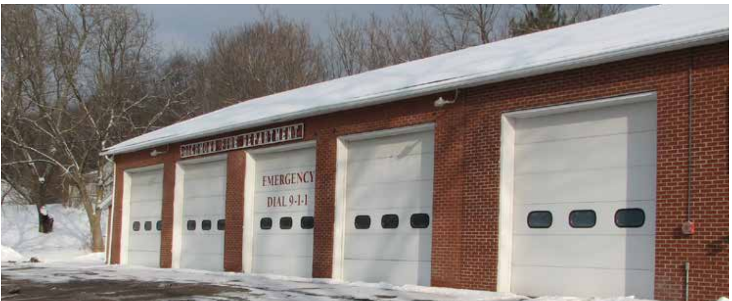
Apparatus Bay overhead doors with inadequate lighting
