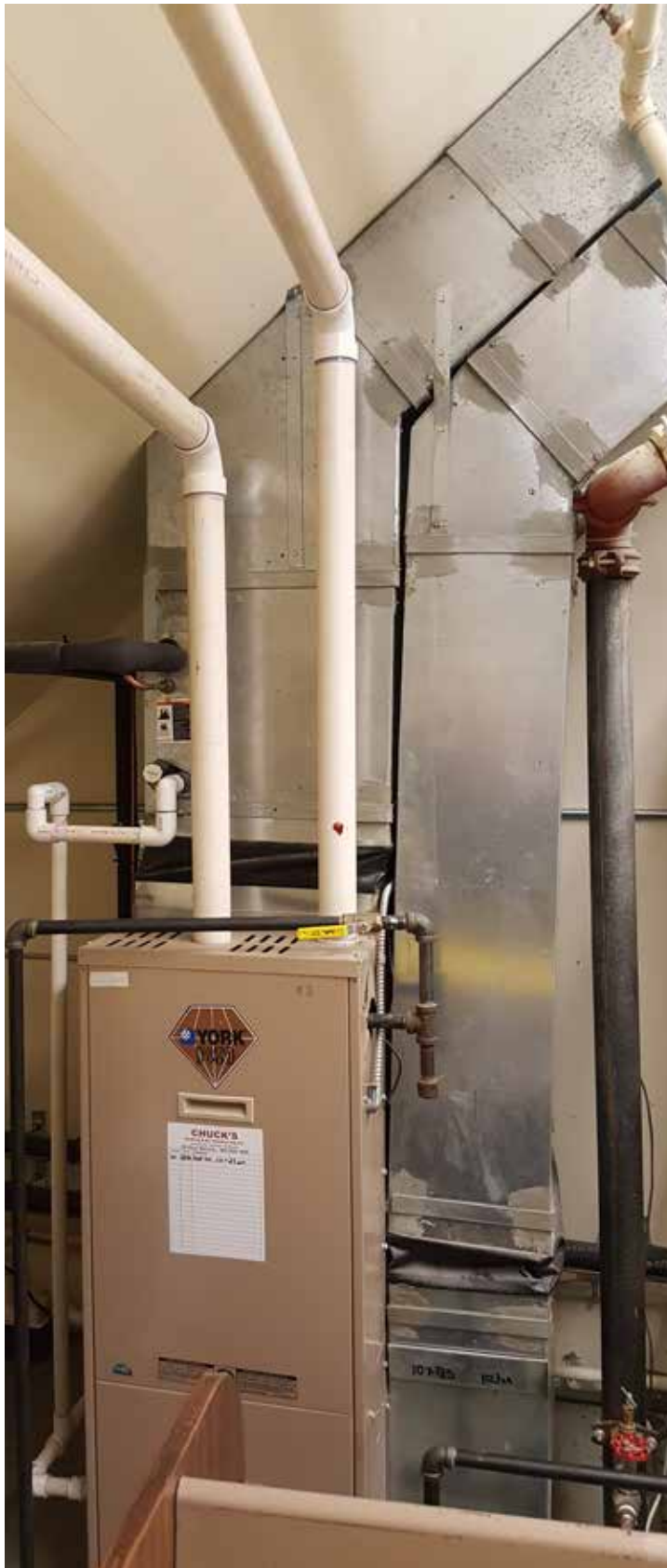
Intake & Exhaust ducts from Outdoor Air Furnaces
