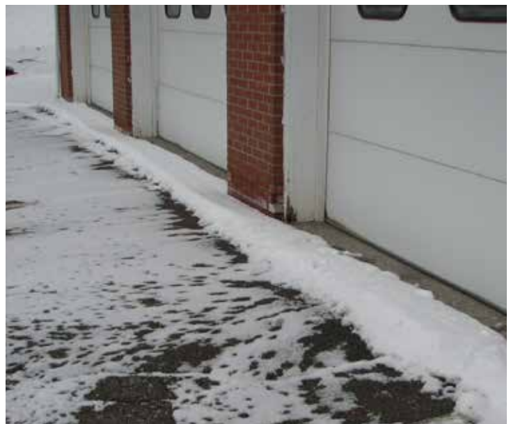
Ice build up at overhead doors
