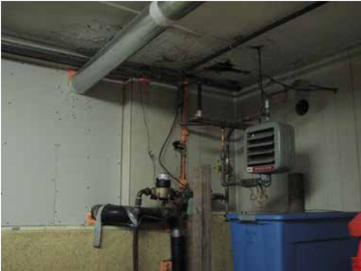
Water service entrance
