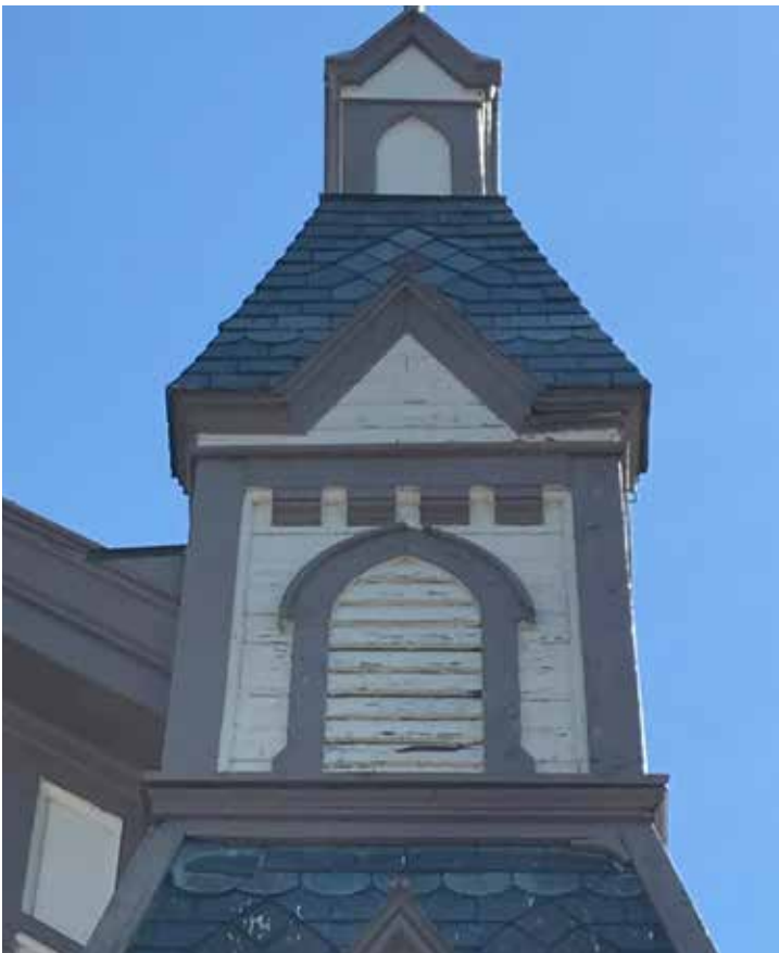
North gable end rot
