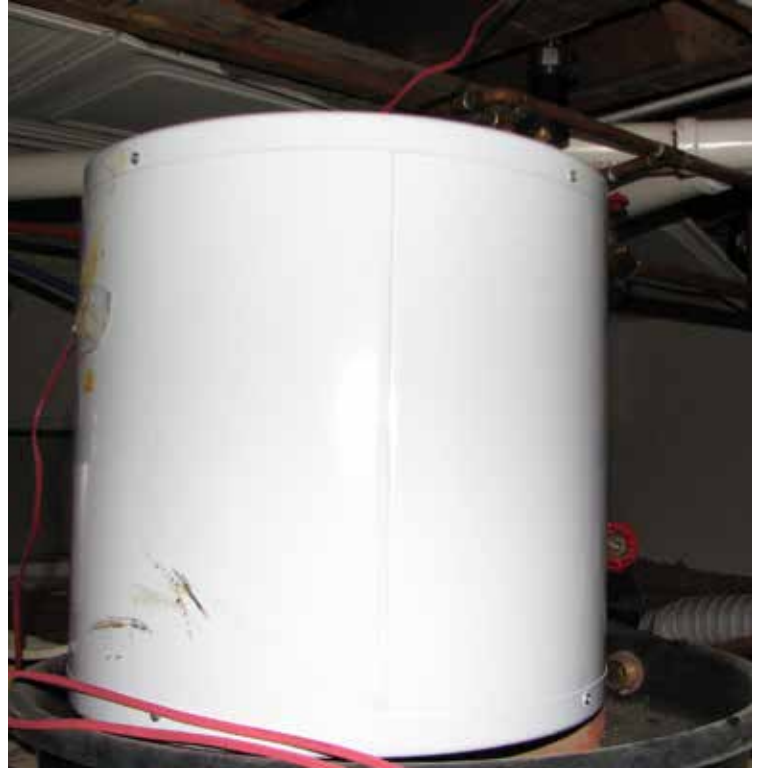
On demand hot water heater above bathroom ceilings
