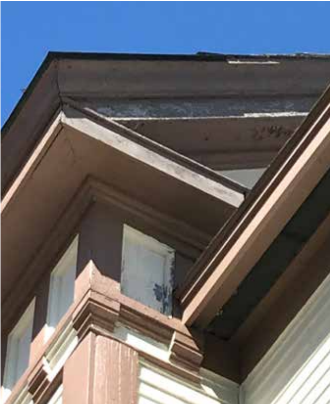
Wood trim rot and peeling paint
