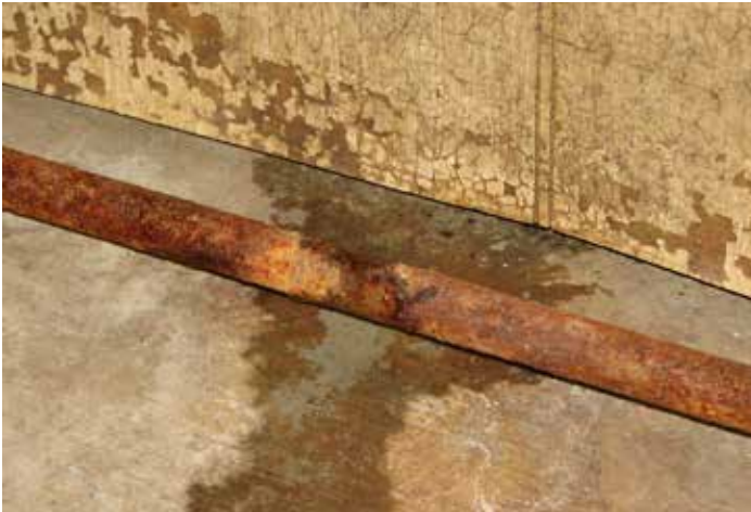
Corrosion of water service pipe
