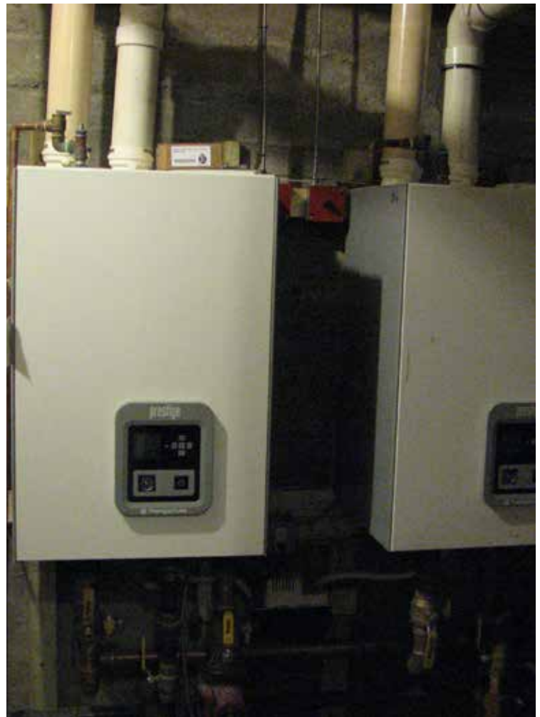
New natural gas, high efficiency boilers in basement
