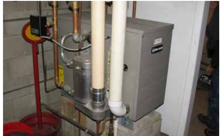
Boiler in apparatus bay
