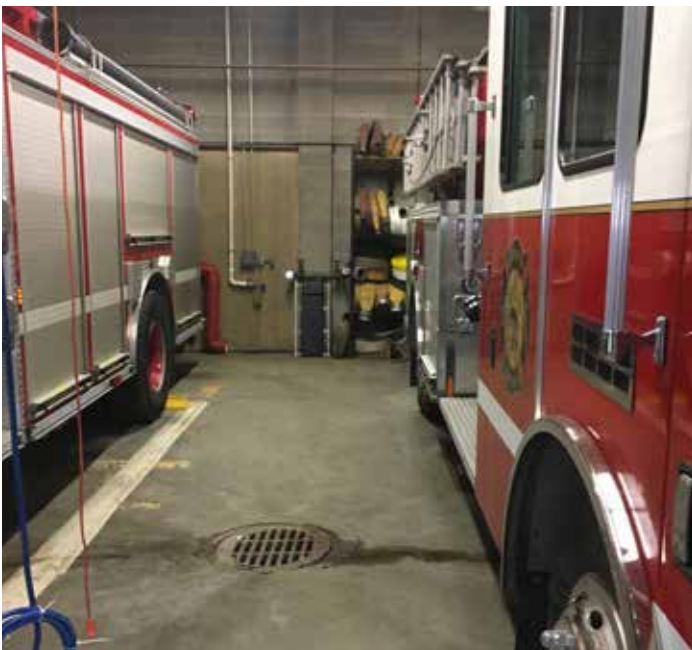
Floor drain in apparatus bay
