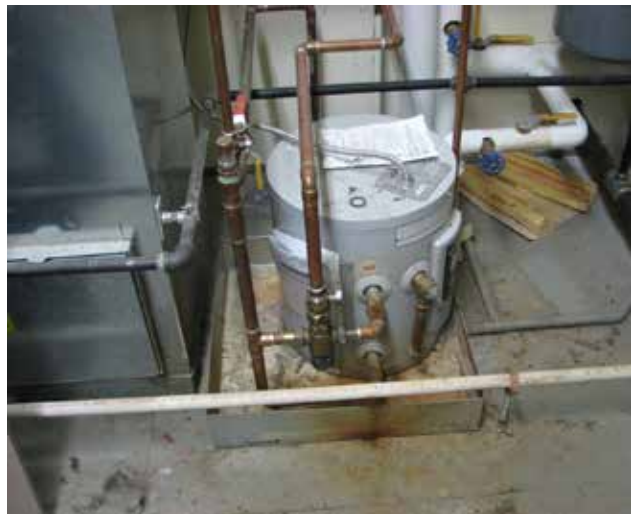
Third floor hot water heater
