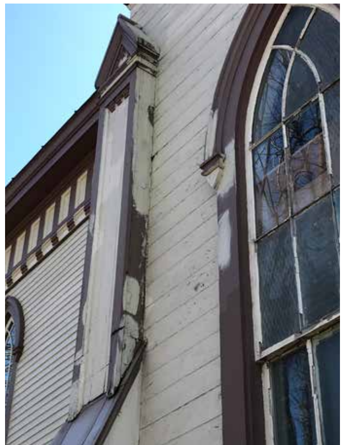
East elevation paint damage
