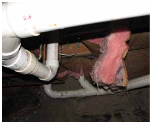
Insulation falling from floor joist cavity
