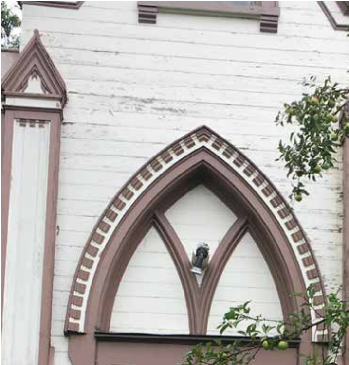
Paint peel and rot at northeast steeple above door
