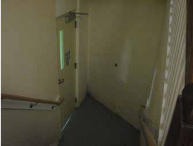
Exit door in lower level cannot open to 90 degrees
