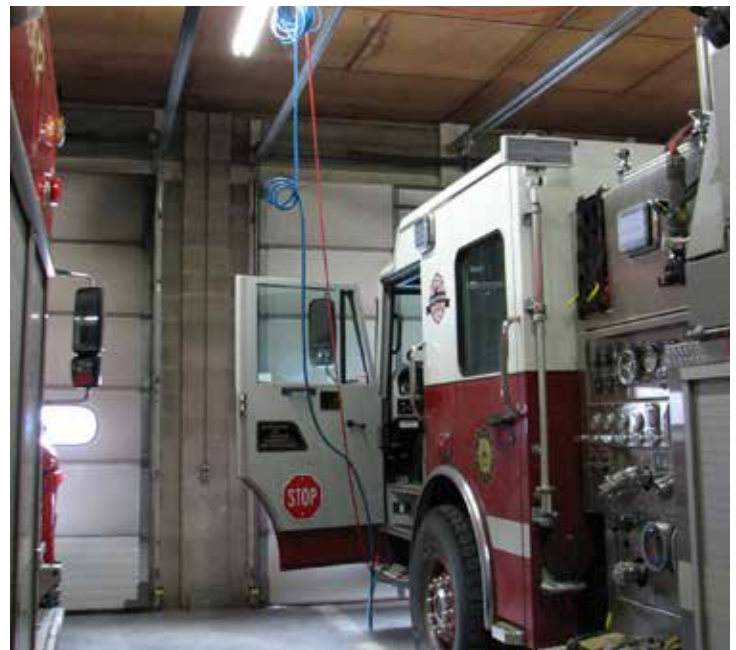
Air and power supply from apparatus bay ceiling
