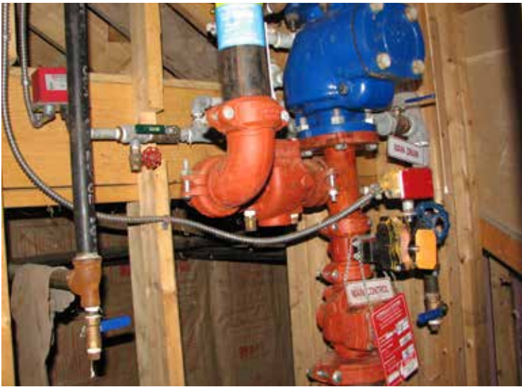
Sprinkler service entrance
