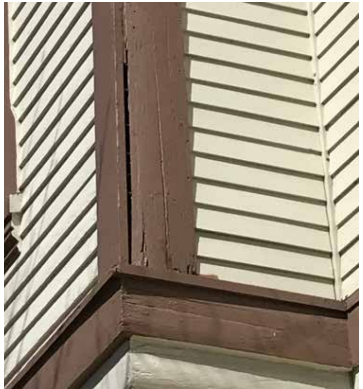
Damaged wood trim
