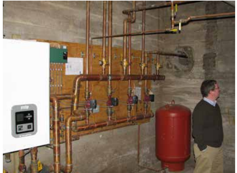
Hot water manifold
