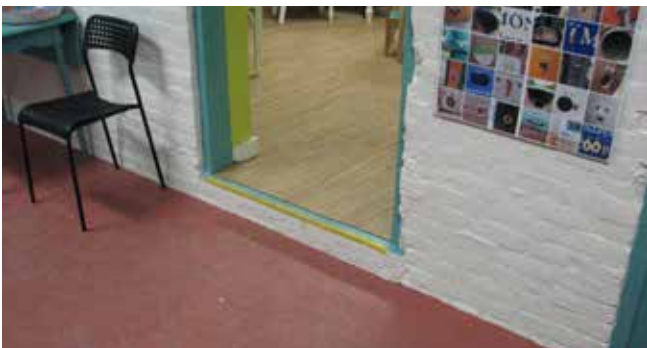
Non ADA accessible classroom space in lower level
