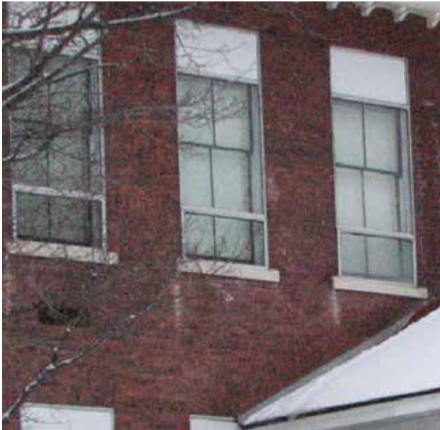
Efflorescence at window sill
