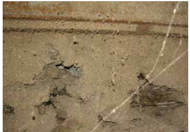
Insulation collapsing at interior of foundation wall
