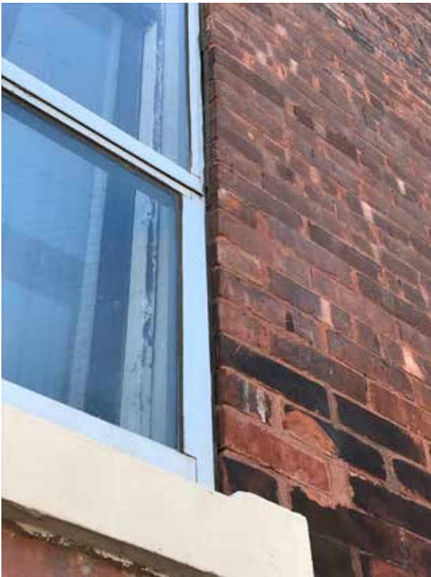
Cracked perimeter caulking at jambs
