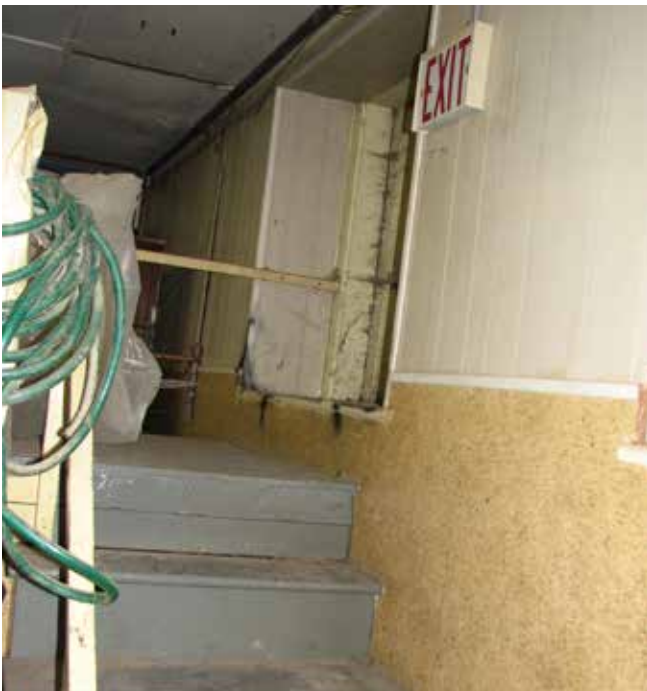
Non compliant egress stair from storage in lower level
