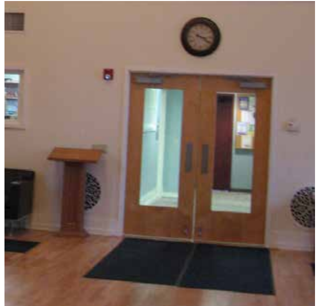
No exit sign at community room doors
