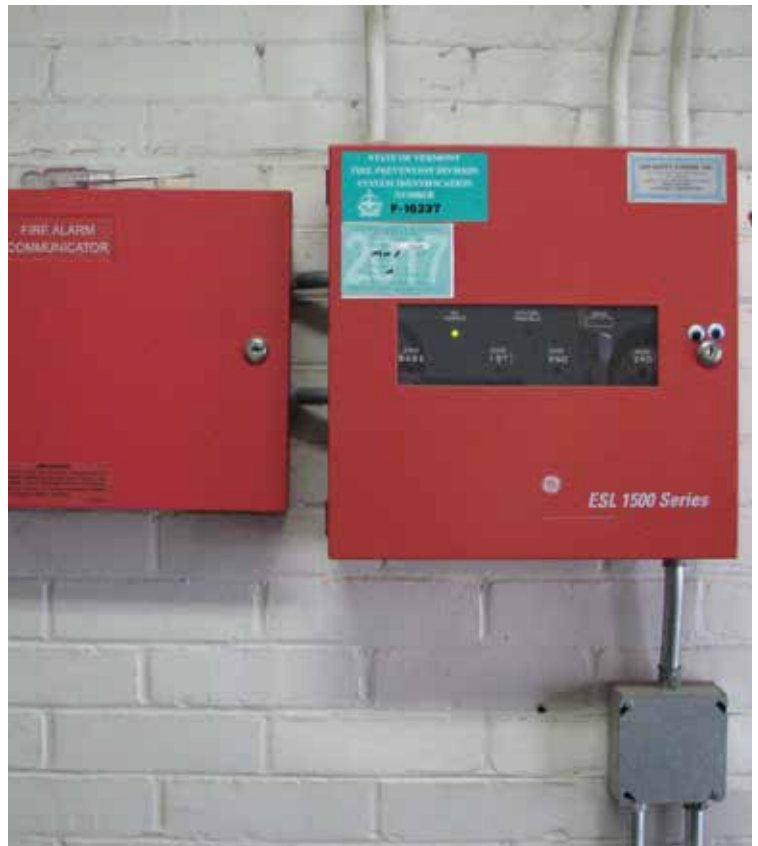
Fire alarm control panel or partial alarm system in entry
