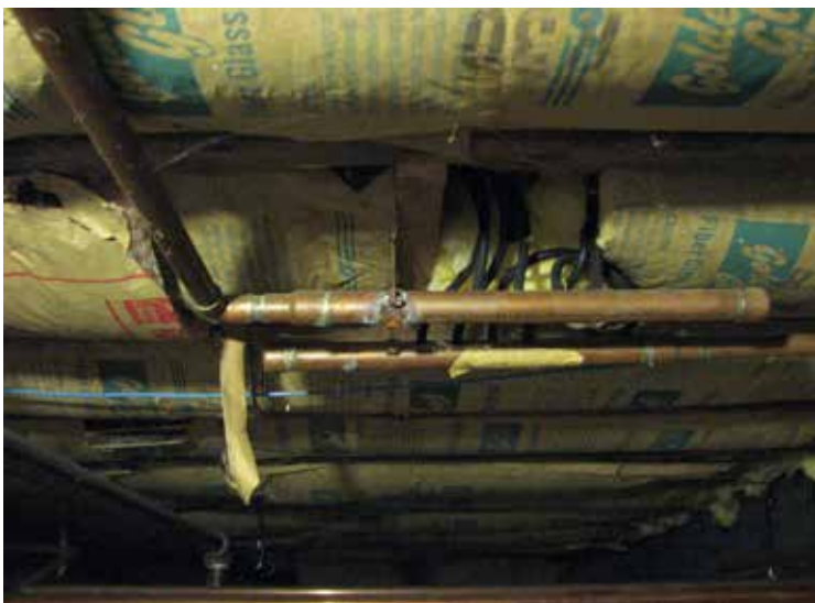
Corrosion of copper piping in radiant floor system
