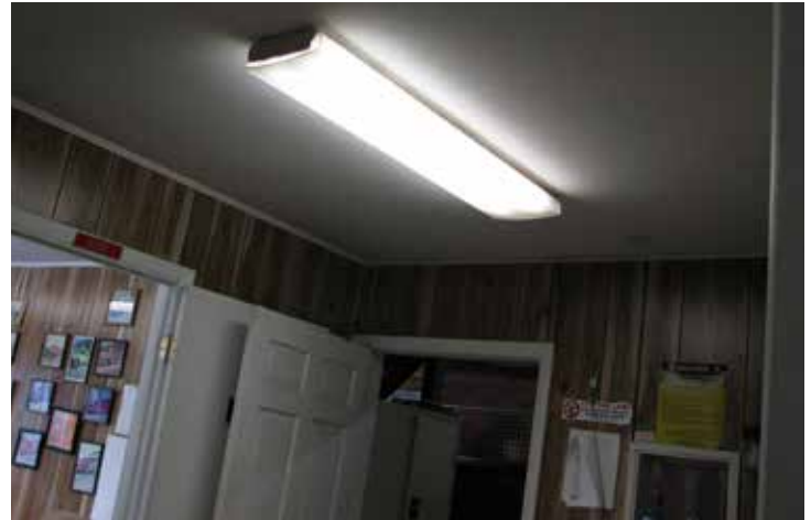
Two-bulb T8 fluorescent light fixtures
