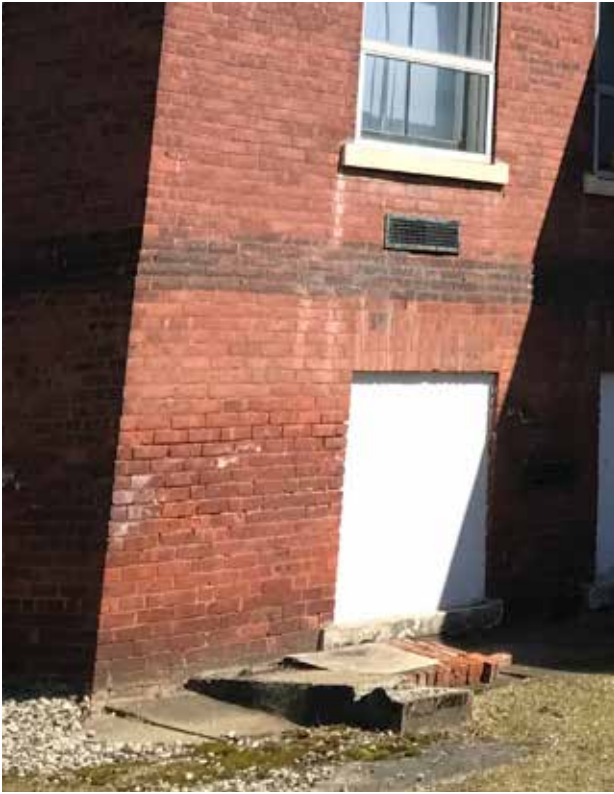
Deteriorating brick mortar at NW corner
