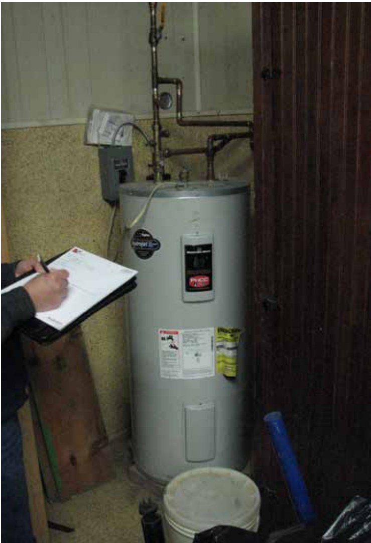
Water heater for Town Office and Post Office domestic
