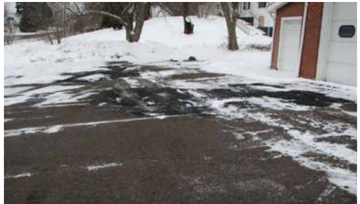
Patched sink hole
