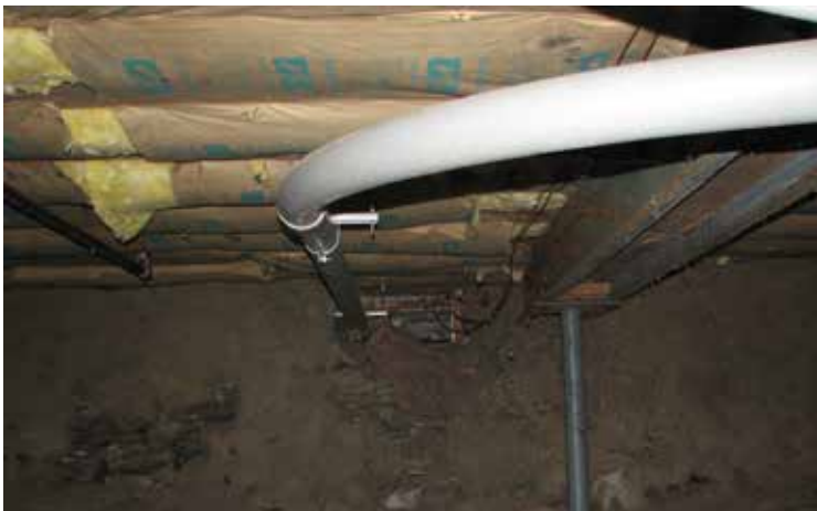
Unsealed pipe penetration through foundation
