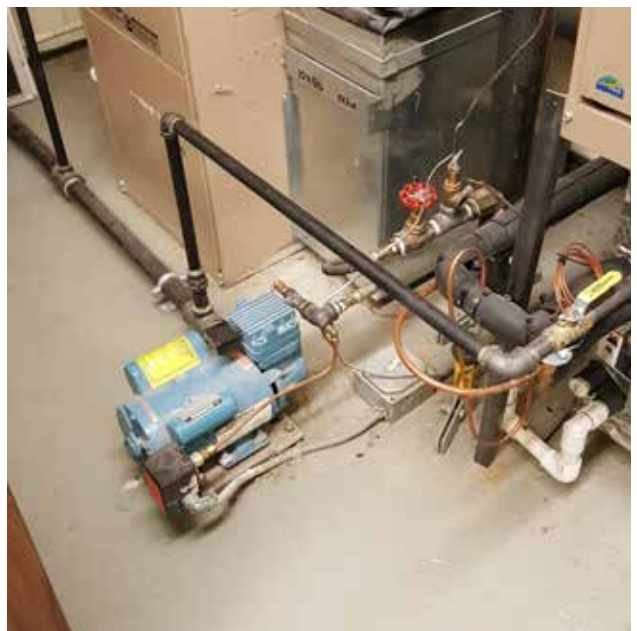
Third Floor Sprinkler system pump
