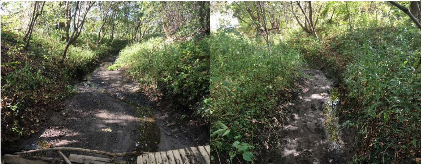
Photo 1. Eroding drainage ditch down-slope of existing outfalls.
