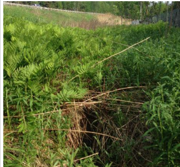
Photo 2. Potential treatment area within the VTrans ROW downslope of culvert outlet. Note erosion in the foreground, which joins gullying from culvert outlet and reaches USD 17 property.
