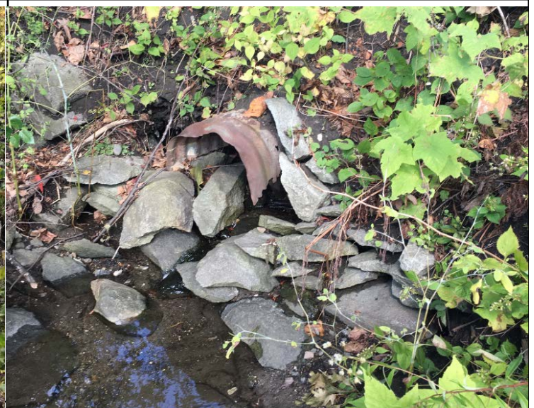
Photo 2. Corroded and undersized culvert
