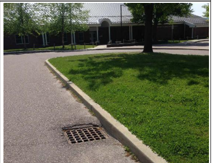
Photo 2. Potential overflow location at existing catch basin.
